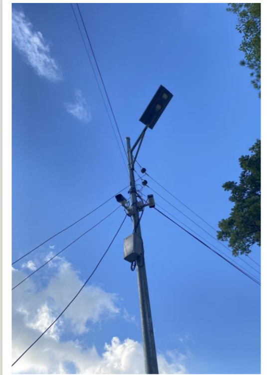
CCTV installed within the campus
